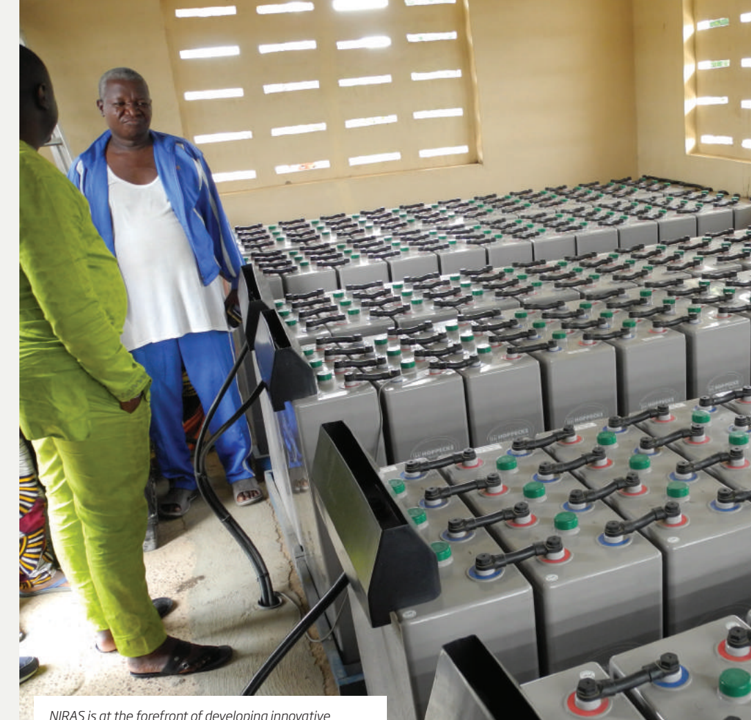
NIRAS is at the forefront of developing innovative energy finance schemes, ensuring the delivery of clean, affordable and sustainable energy to the world's poorest people. Pictured here: energy storage batteries for mini solar power plants at Grand Popo, Benin.
